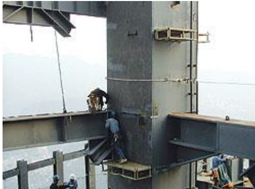
Erecting and welding steel columns was major challenge. (Photo courtesy of Turner International)
