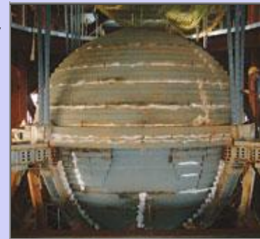
Tower's tuned mass damper was assembled on site from 12-cm-thick steel plate.
