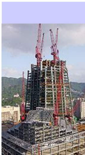
Lower floor megacolumns slope inward with the building's facade. (Photo courtesy of Turner International)
